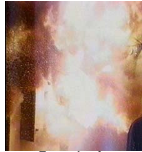
Example of an arcing fault
