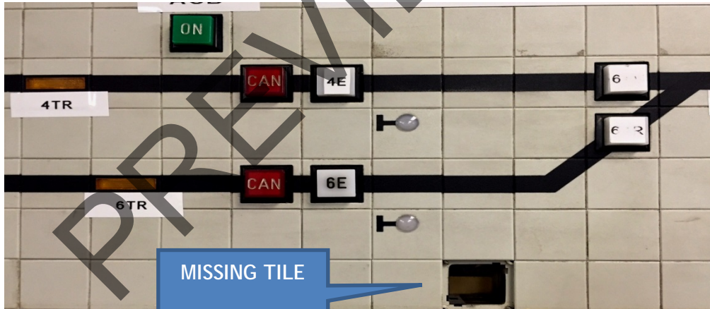
Figure 2.3 Missing Control Panel Tile
