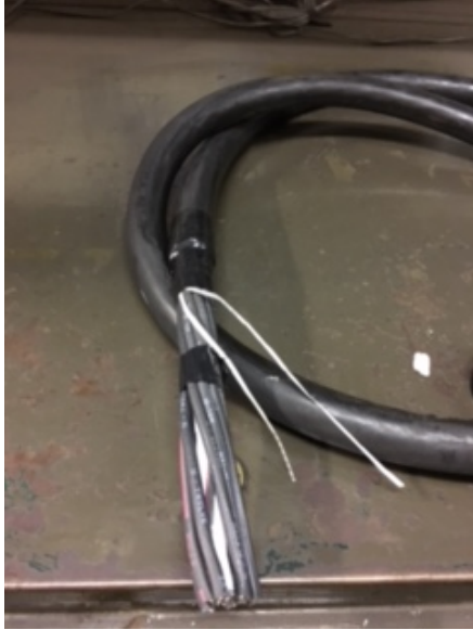
Figure 2.11 Typical Signal Cable
