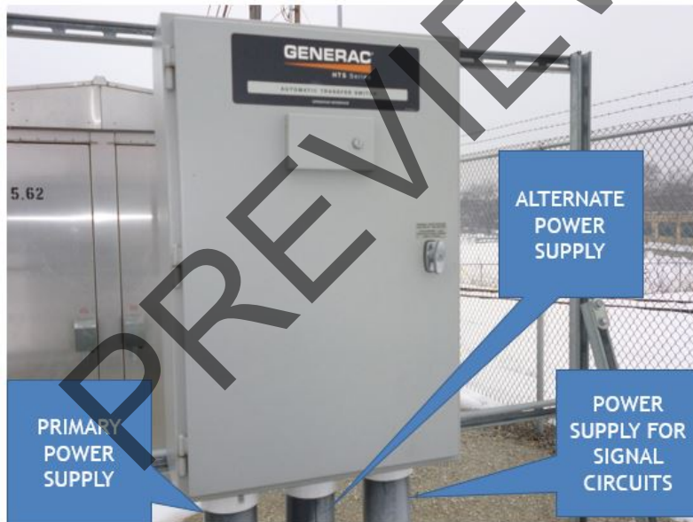
Figure 2.2 Primary Power at the Automatic Transfer Panel
