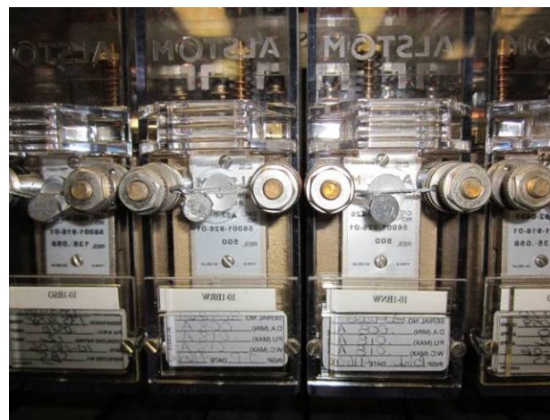
Figure 4.2 A Group of Alstom B1 Relays - Courtesy MBTA
