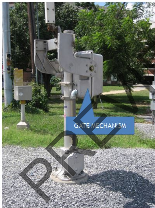
Figure 17 Gate Mechanism at a Highway Grade Crossing
