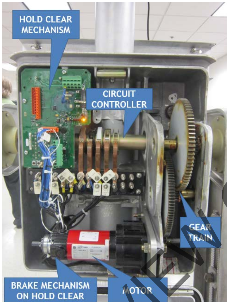
Figure 20 Safetran S60 Gate Mechanism Circa Approximately 2005
