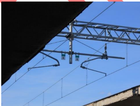
Figure 4 Overhead Contact system
