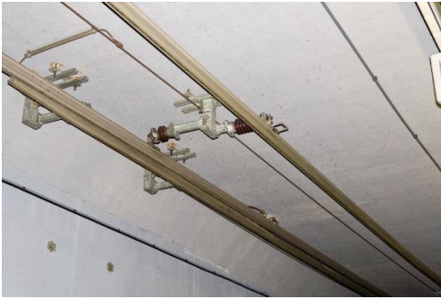
Figure 6 Rigid Overhead Conductor System
