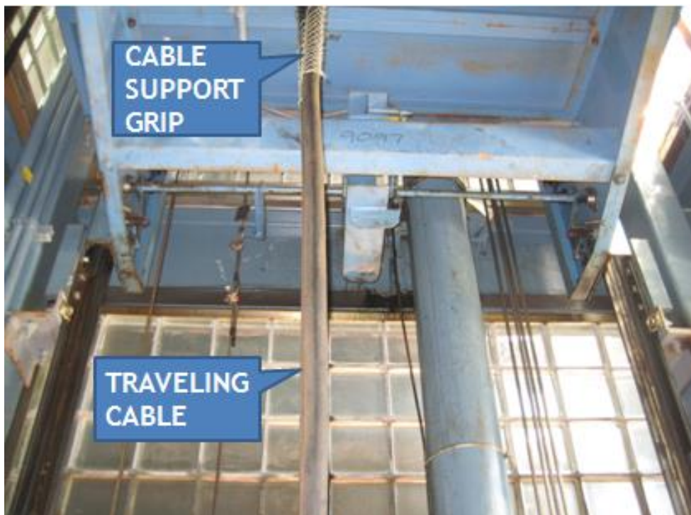
Figure 4.9 Traveling Cable in a Transit Hydraulic Elevator System –Courtesy NYCT
