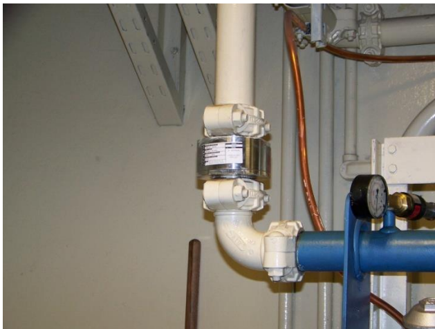
Figure 2.6 Isolation Coupling Installed Between the Power Unit and Hydraulic Cylinder –Courtesy NYCT
