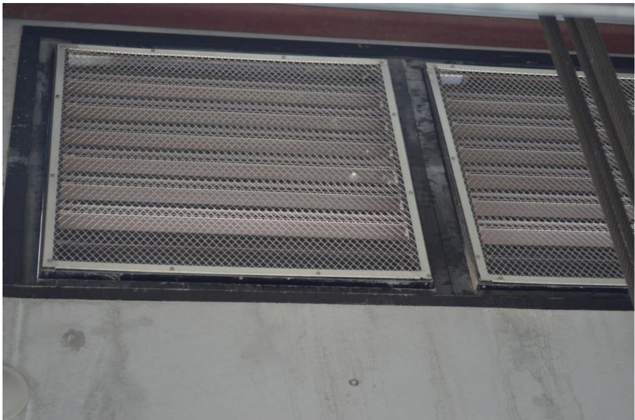
Figure 4.2 Hoistway Vent –Courtesy WMATA
