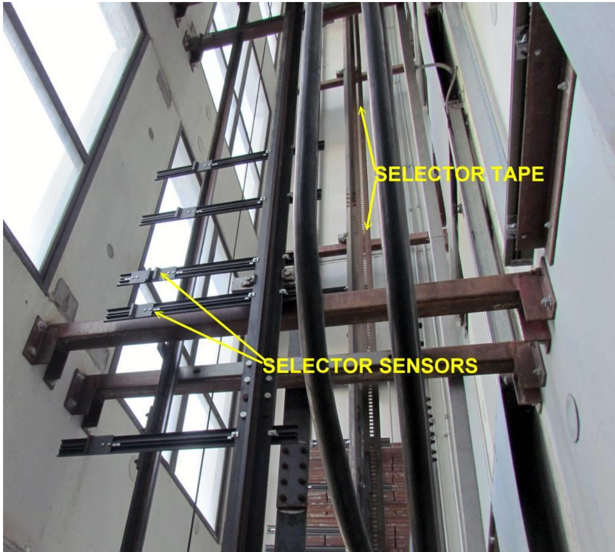
Figure 3.8 Selector Tape and Sensors in Hoistway –Courtesy WMATA
