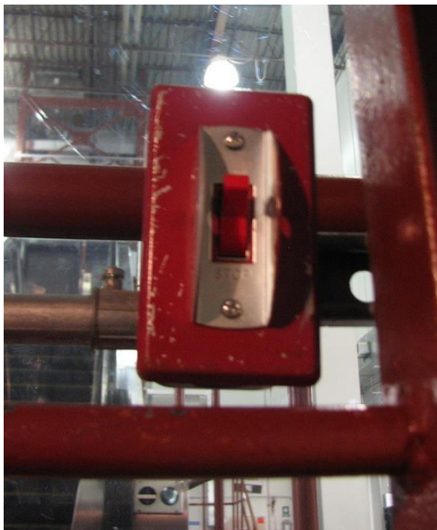
Figure 4.22 Pit stop switch –Courtesy WMATA
