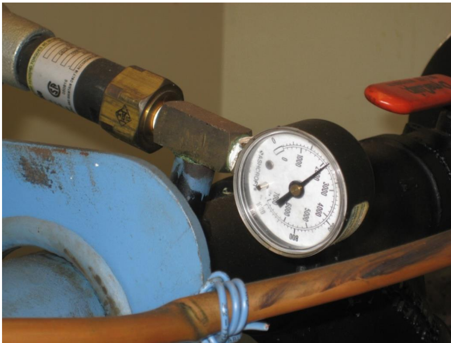
Figure 2.3 Pressure Gauge with Pressure Switch –Courtesy NYCT
