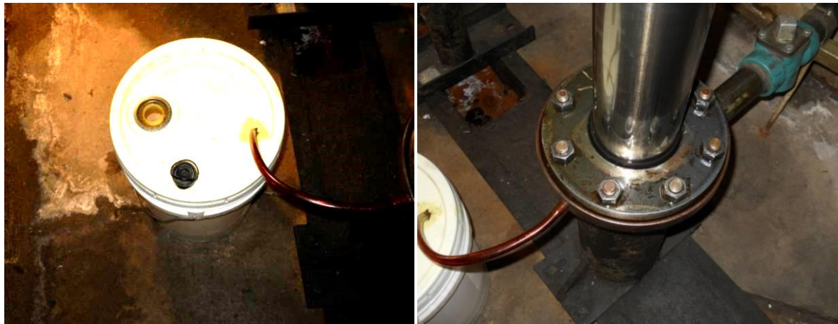
Figure 1.2 Used Five Gallon Bucket used as a Catch Basin for Hydraulic Elevator –Courtesy WMATA
