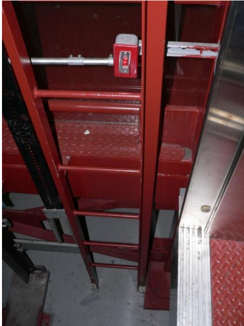
Figure 4.21 Pit Ladder -- Courtesy WMATA
