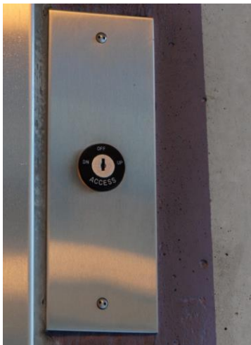
Figure 3.6 Independent Control Key-Switch - ©Elevator Bob
