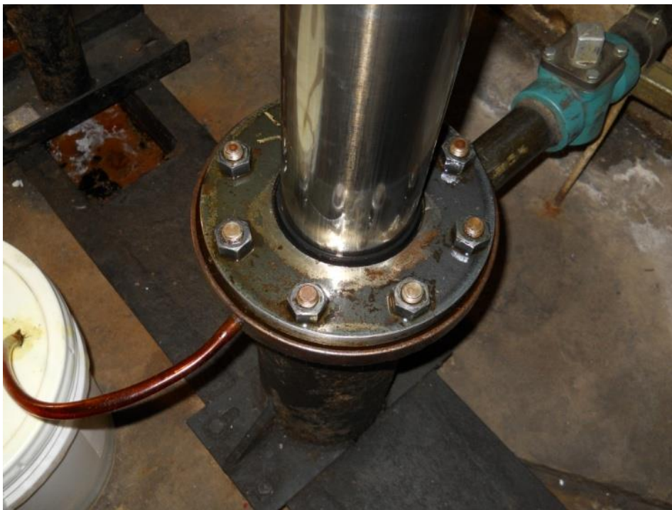
Figure 2.9 Bucket Style Scavenger –Courtesy WMATA
