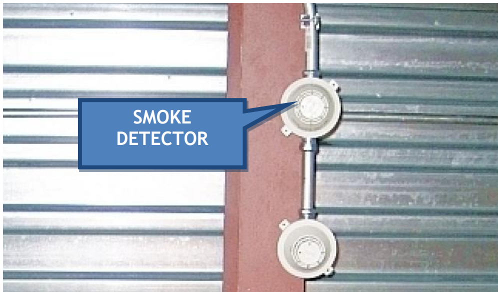
Figure 4.5 Smoke detector located in hoistway
