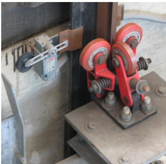
Figure 4.25 Roller guide on guide rail –Courtesy NYCT
