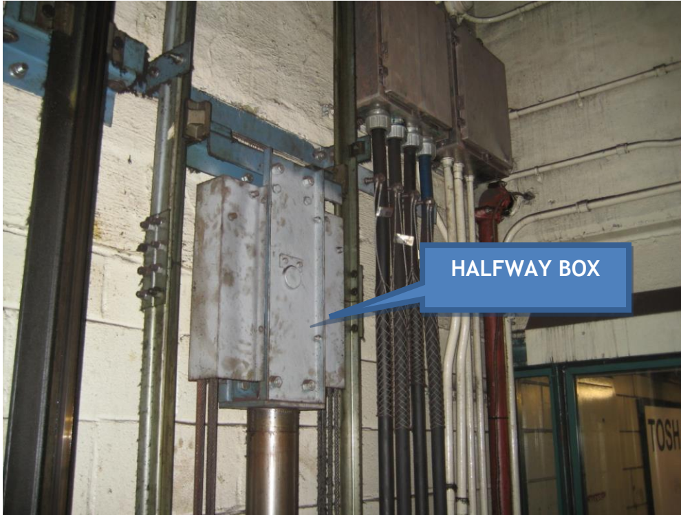
Figure 4.10 Halfway Box –Courtesy NYCT
