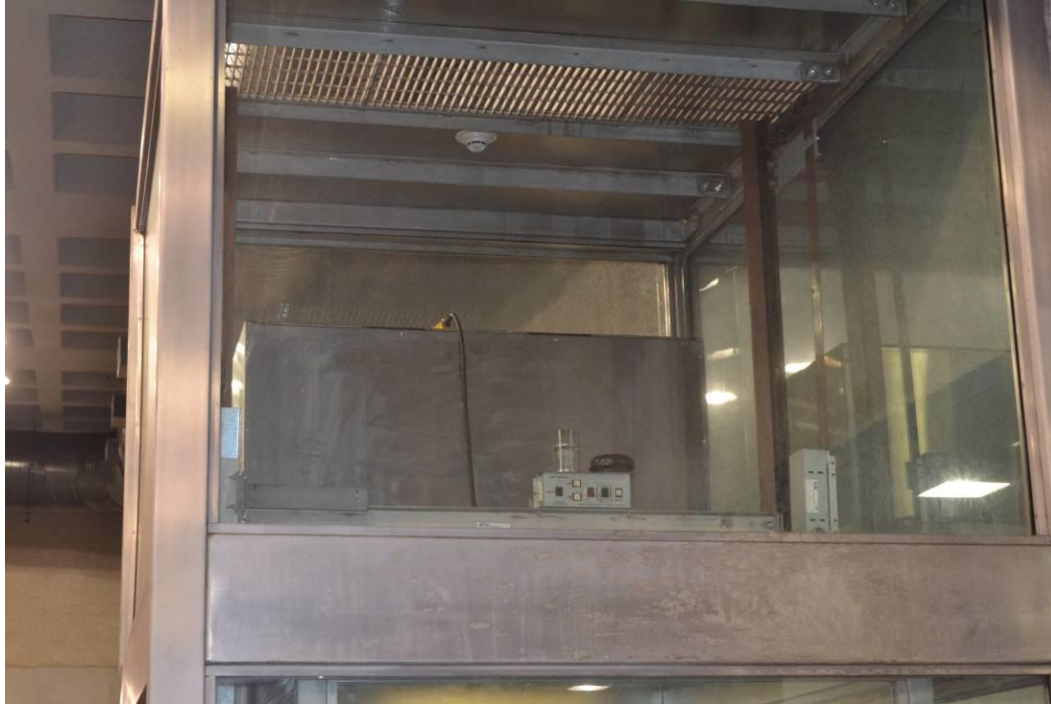
Figure 1.3 Limited Space in the Overhead –Courtesy WMATA
