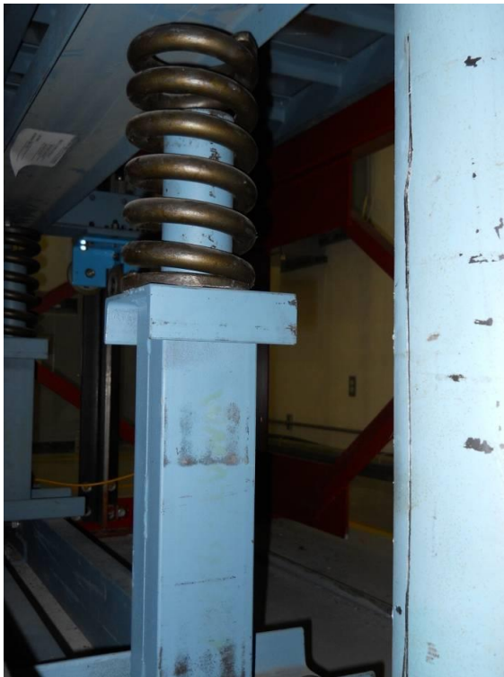
Figure 1.9 Elevator Car on Buffer – Courtesy WMATA
