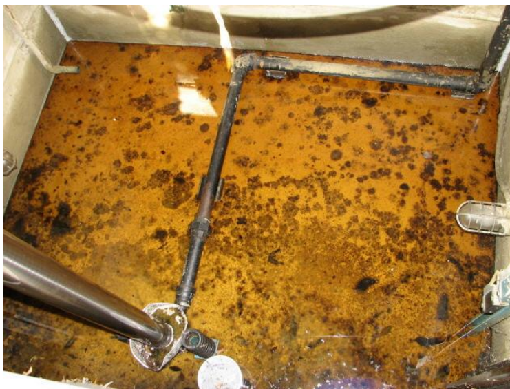
Figure 1.8 Flooded Pit Area ©Elevator Bob
