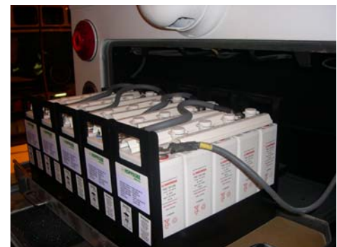
Individual cell transit battery in a battery tray
