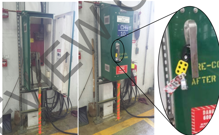
Figure 1.17 Electrical Cutout Box with Lock (Courtesy of MBTA)
